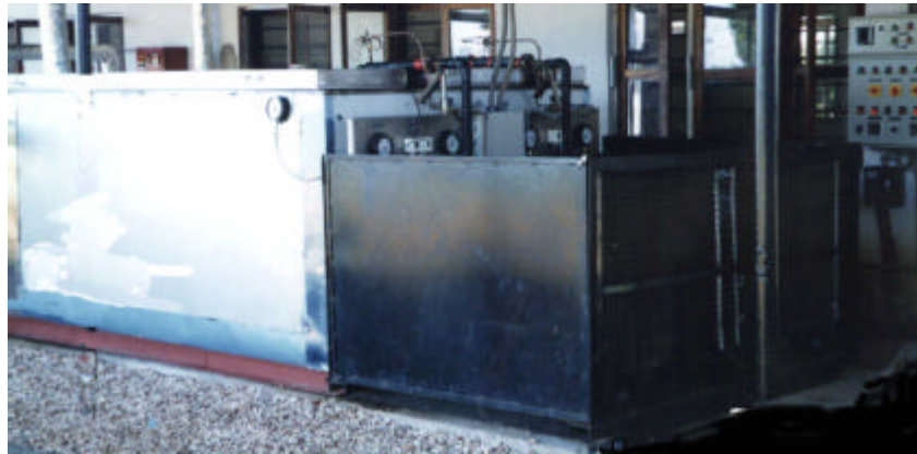
Ice Bank Tank with Refrigeration Unit
