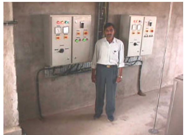
Power Control Panel
